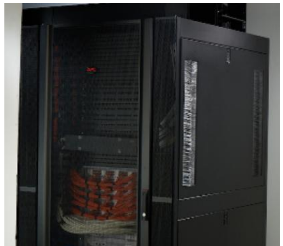
Installed on AR3340 enclosure
